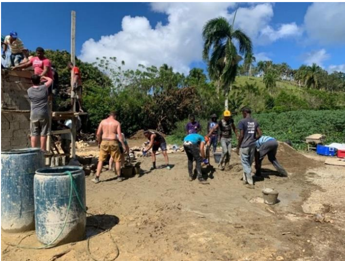
Photo shows group mixing cement for the second floor of the recording studio. Above and to the right shows the yucca garden with prayer mountain behind it.
